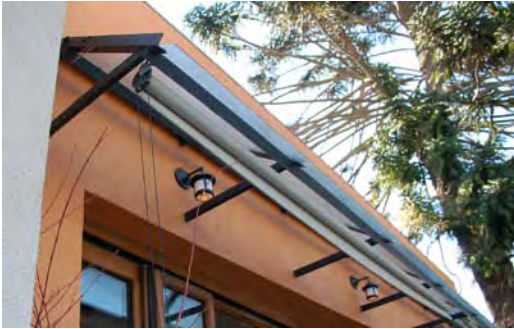
Sconce lighting accents the building architecture.
